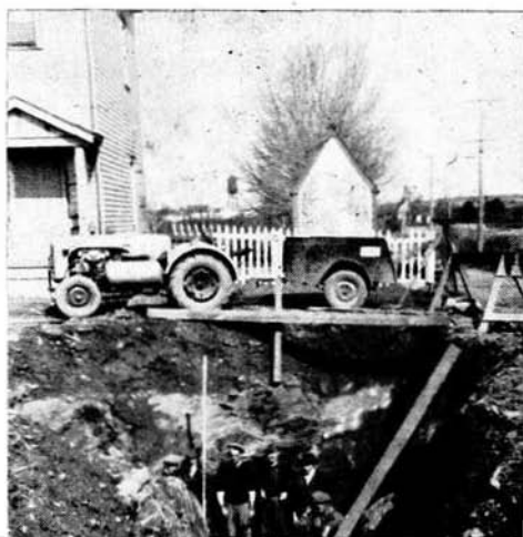
Laying water and sewer mains at Victoria and Boland Road. Note depth and quantity of rock
