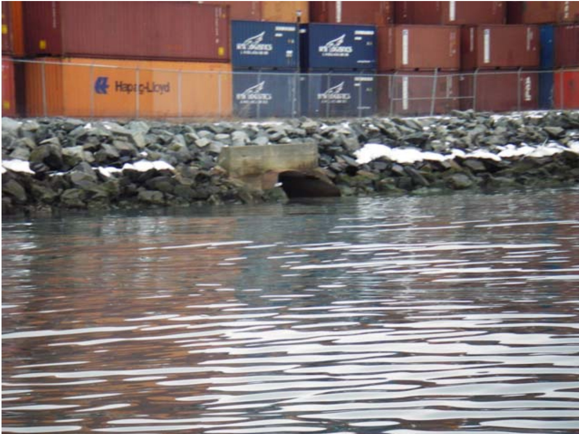
Figure 10. Fairview Cove combined sewer overflow (CSO) from sample site.
