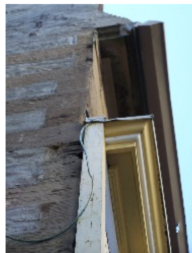
Gaps between masonry corners and storefront trim
