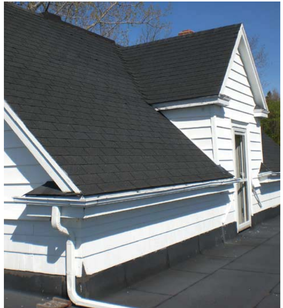
2014 View showing roof cornice return and dormer with door to roof of stone verandah
