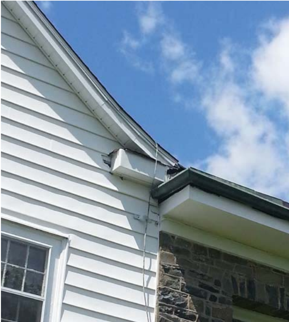
2014 View showing curved roofline of 1942 addition cut off by stone verandah. Some attempt at a cornice return.
