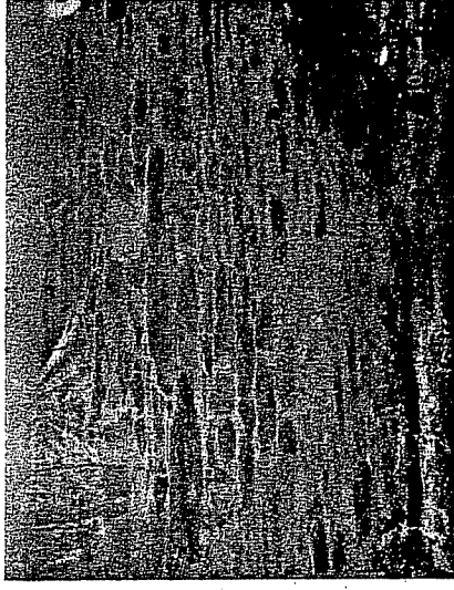
CRACK IN NORTH FOUND BRACKET
