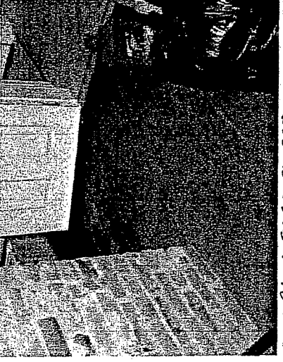
MOLD IN BELOW FLOOR SINK @ KITCHEN 4/82
