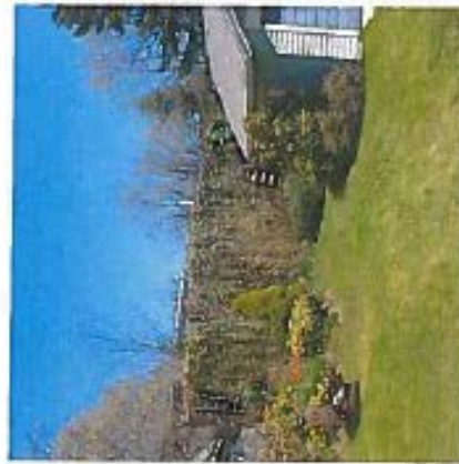
Back wall of shed covered with ivy, before demolition, from Seldon Street side
