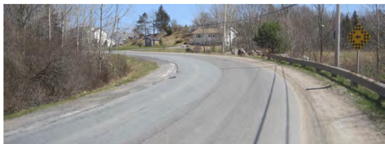
Photo 2 - Looking east on Walker Service Road towards Old Sackville Road from the proposed site Driveway. Visibility to and from the east can be improved by removing bushes on the inside of the curve at the left side of the photo.
