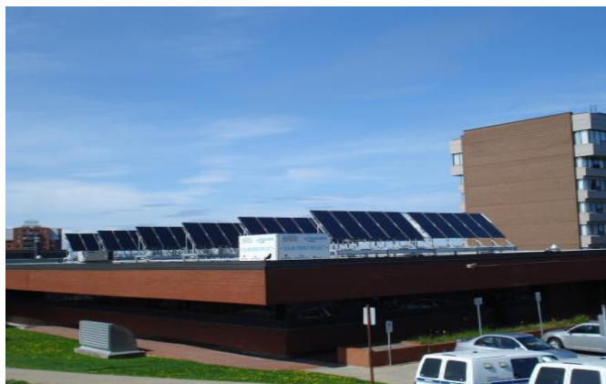
Halifax Police Station utilizing solar hot water
