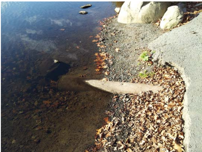
Photo 1 – Oathill Crescent Storm Sewer
