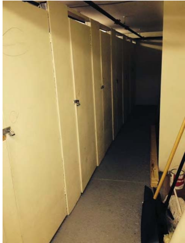
Figure 2 - Photo of area in building where three additional units would be created through internal conversion.
