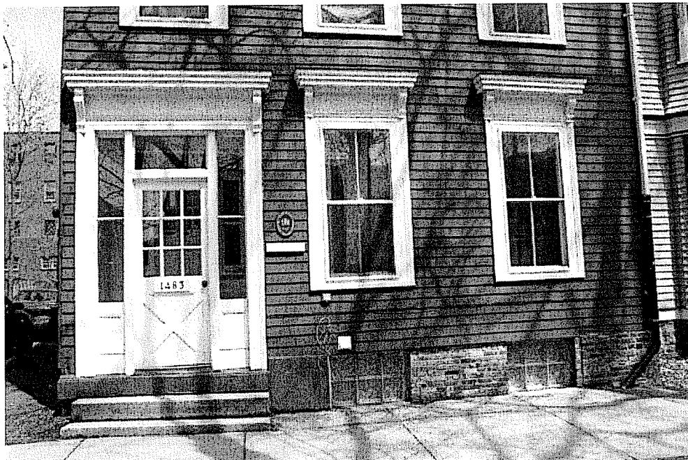
Front elevation of 1483 Carlton Street showing glass block in place of the basement windows.
