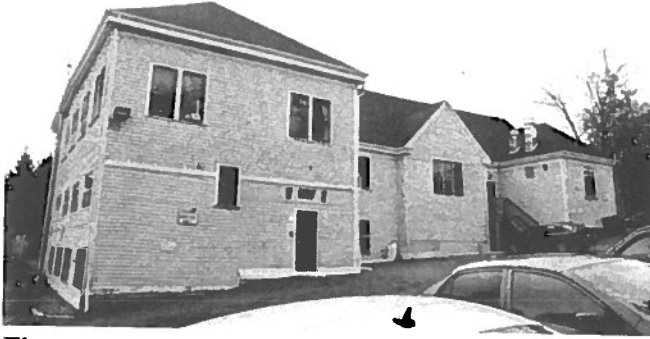
Figure 1: North Elevation – the original building including two cross gables with hip and gable roofs (right) and the historic three storey addition with hip roof (left)
