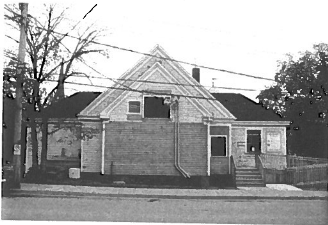
Figure 3: West Elevation – The red brick chimney and two windows on the cross gable with hip roof will be removed
