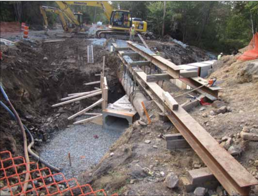
New stormwater box culvert installed under existing water transmission mains at Coronet Ave. , Halifax
