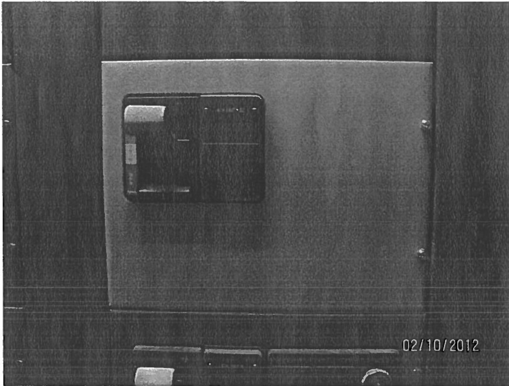
MCC Cabinet – East Ice Level Mechanical Room
