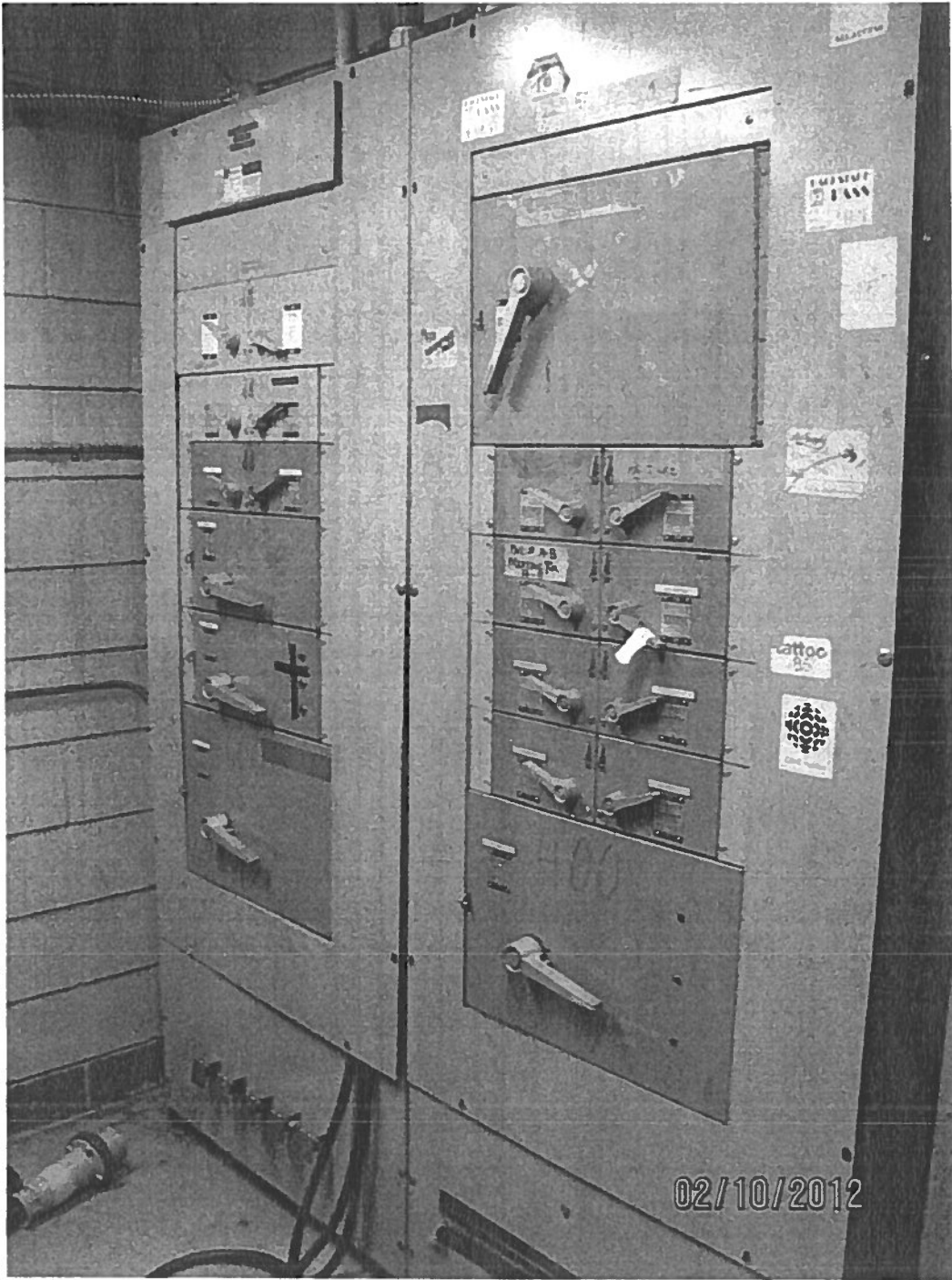
Entertainment MCC – North Level 97 Electrical Room
