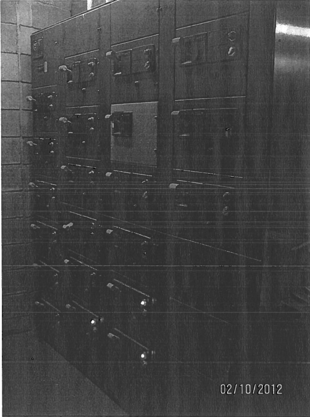
MCC Cabinet – East Ice Level Mechanical Room
