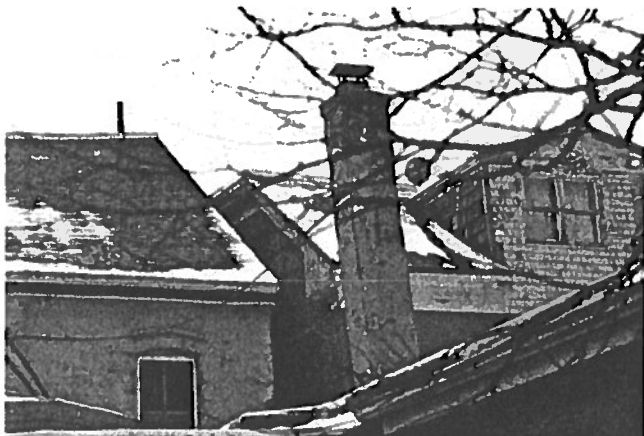
Figure 3: Rear window to be altered and red brick chimney to be removed from the original rear ell
