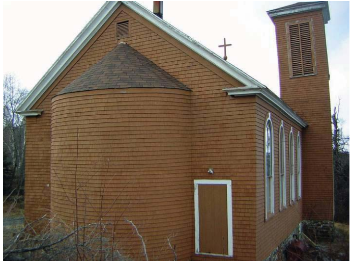
Figure 4: Rear and harbour side of the church building showing the apse, framed window openings, and the tower.
