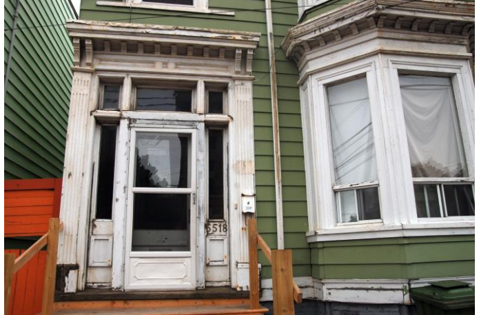
Figure 2: The building includes Italianate features such as the bracketed cornice and two-storey bay window as well as classical features such as the decorative trim on the front door
